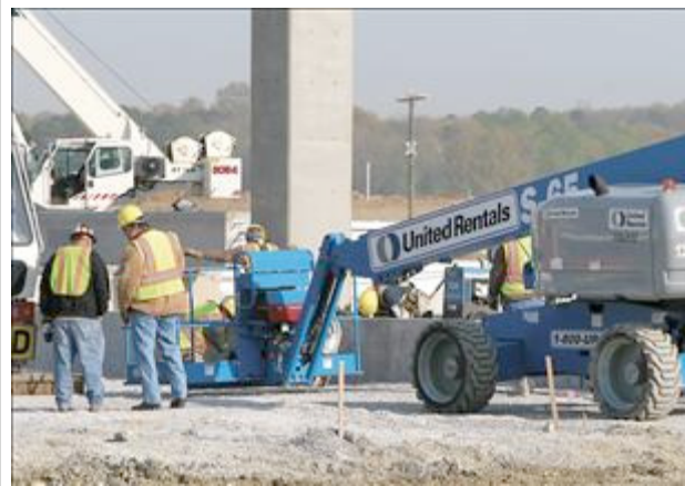
Staff Photo by Dan Henry Workers check the first concrete beam installed at the new Volkswagen group assembly and paint shop site..
